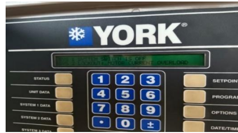
Gambar 2 Alarm Chiller motor current overload
