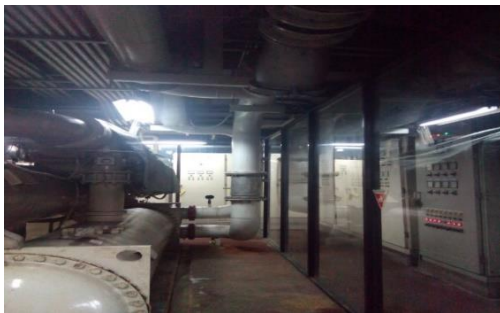
Gambar 1. Ruang Panel Chiller
